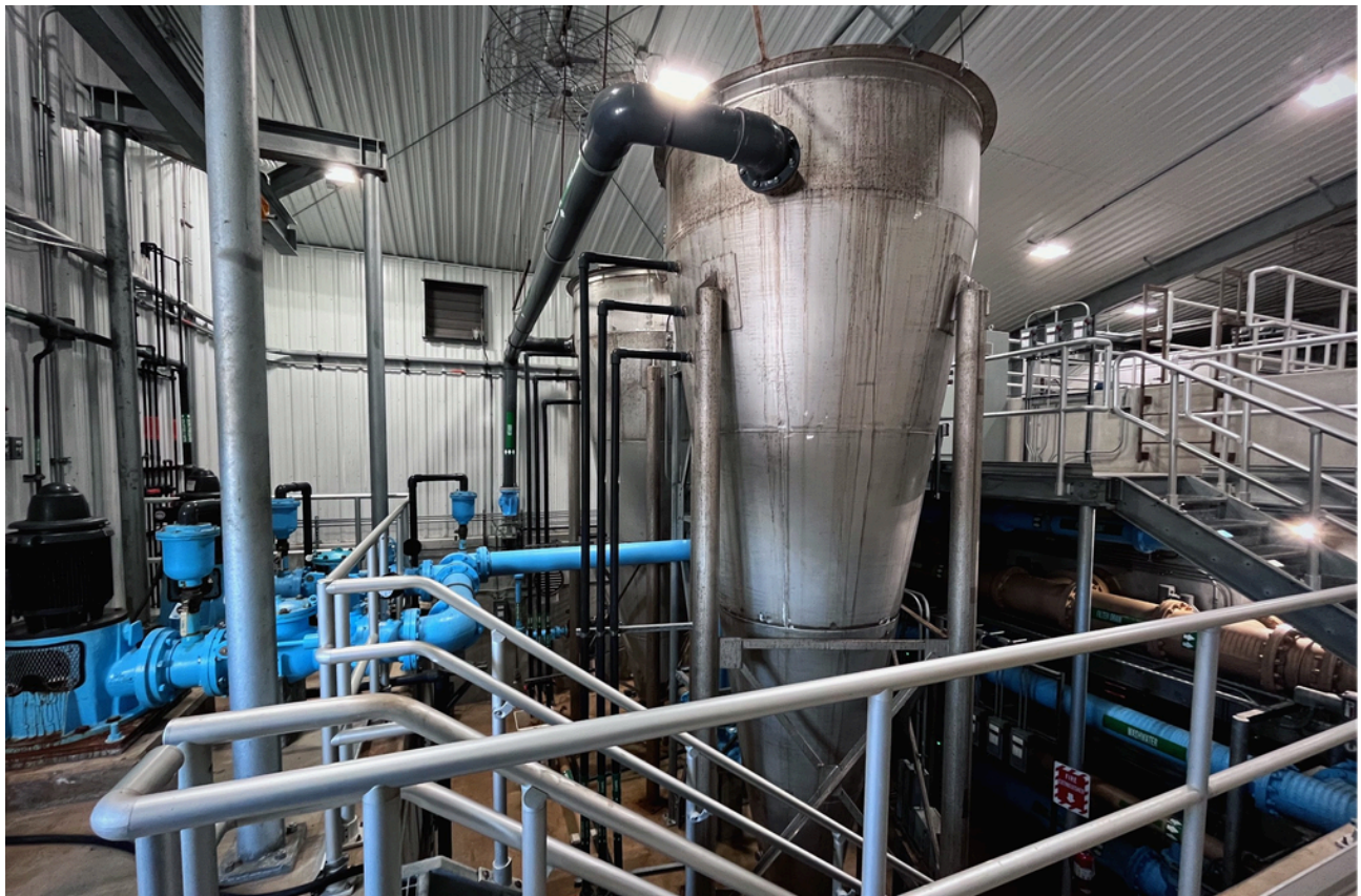
Water filtration at the Water Treatment Plant.
